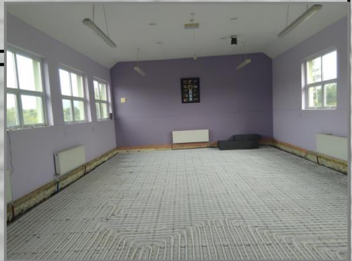
Above: Deployment of ThinICE™ radiant floor in Mayo demonstration building
