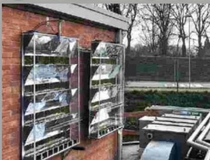
Above: Deployment of CPC-PCM PVT panels, Ferrara, Italy
