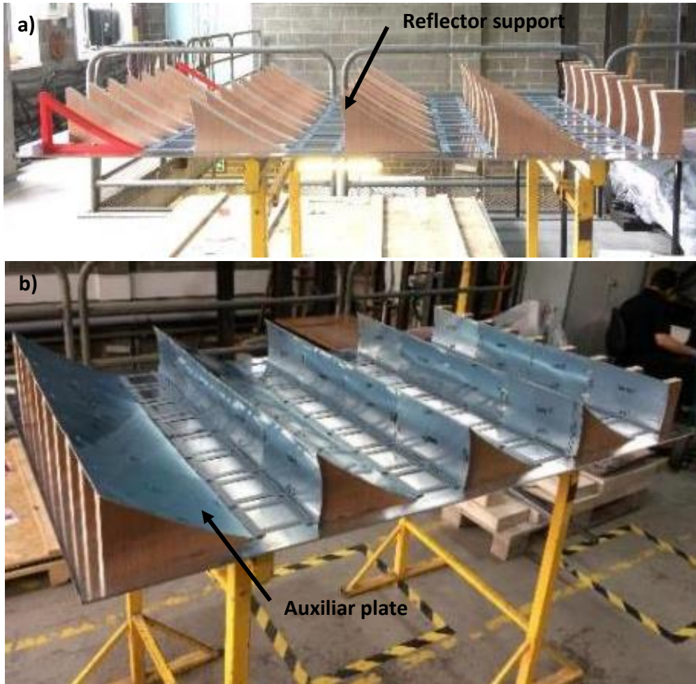
Figure 6. 15 (a) Reflector supports installed on the backplate (b) Final installation of the reflector supports with the auxiliary plate
